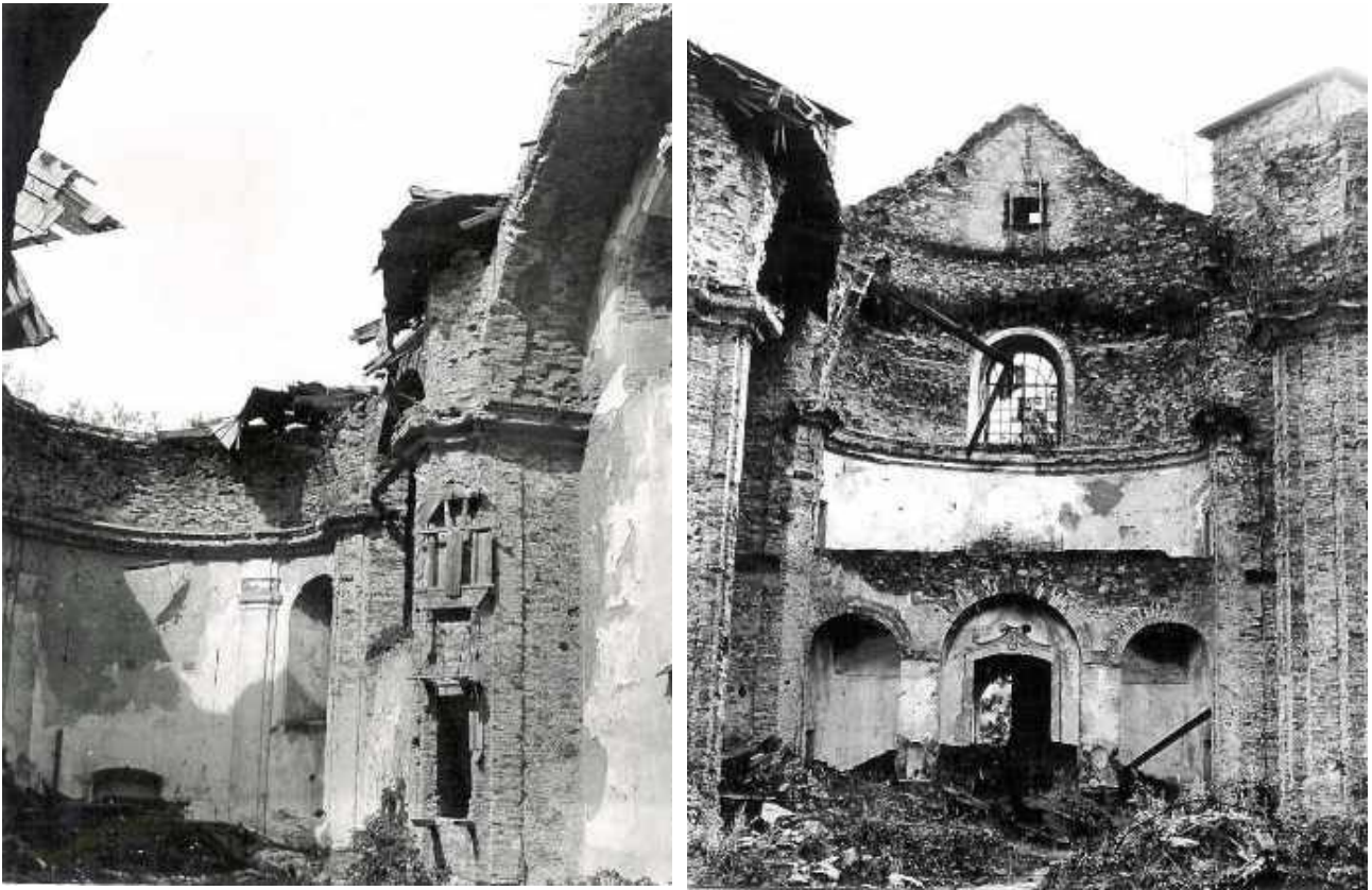
A view to the altar and main entrance after the fall of the roof at the end of 1960's . Photo shows the condition in 1972.
